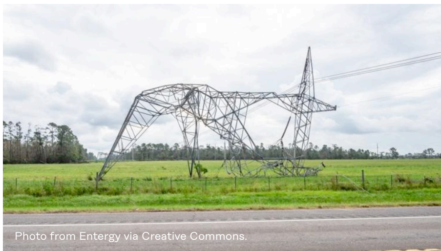
Figure 9. Damage from Hurricane Laura on overhead transmission
