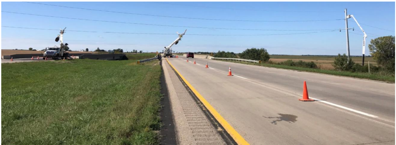
Using boom trucks with bat wings for freeway crossing (photo courtesy of the Wisconsin Department of Transportation Transmission Playbook: Accommodation on Interstate and Freeway Right-of-Way)
