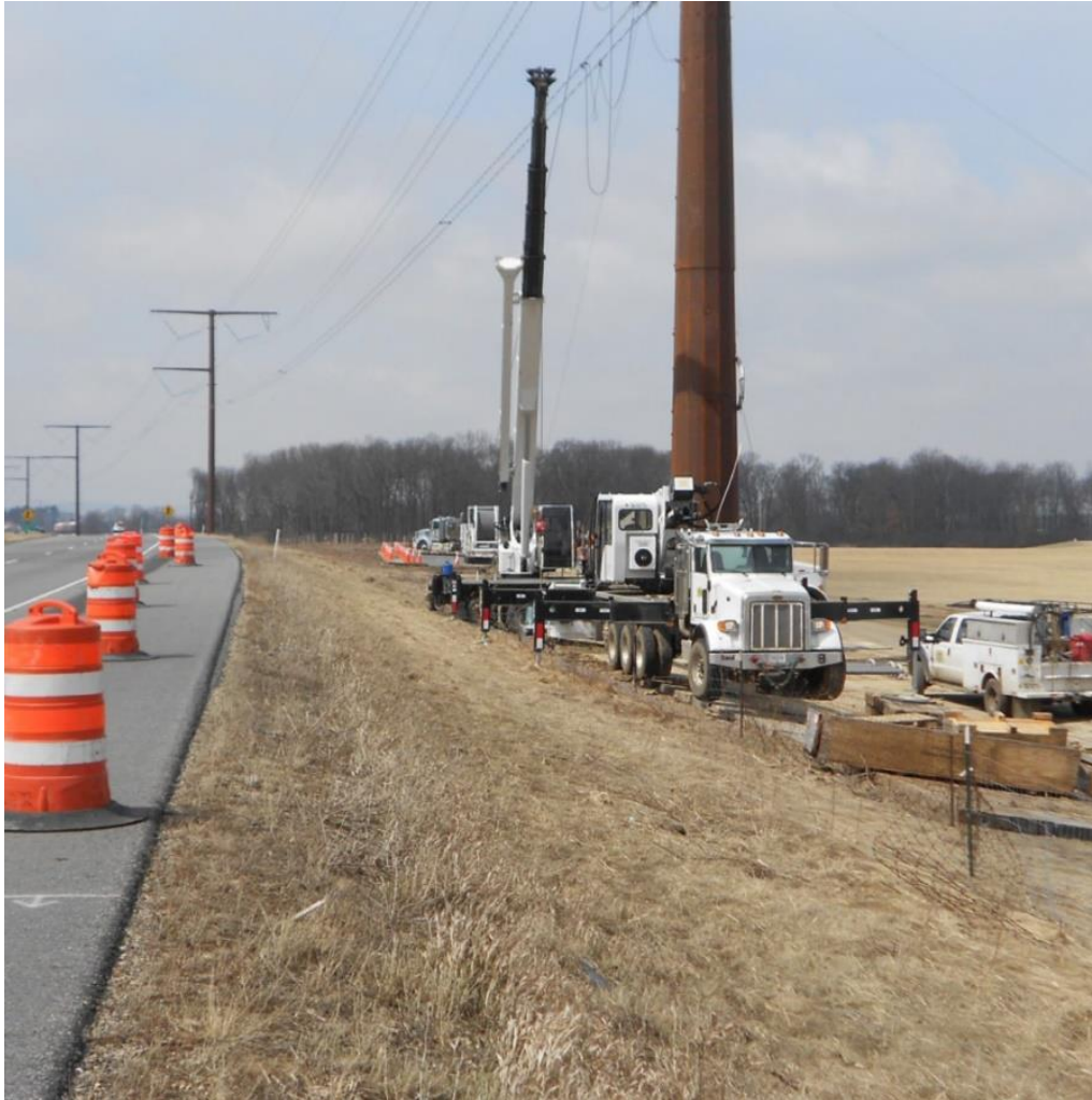
0/94, ATC Badger-Coulee (photo courtesy of the Wisconsin Department of Transportation Transmission Playbook: Accommodation on Interstate and Freeway Right-of-Way)
