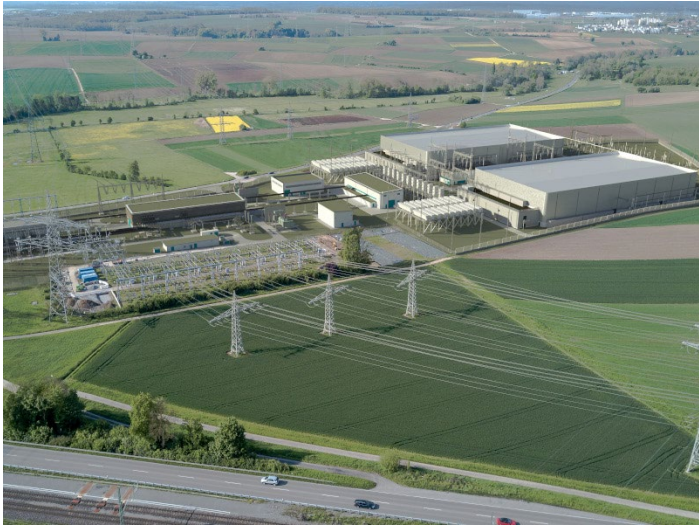
Photograph from NS Energy, “SuedLink HVDC Power Transmission Project.”
